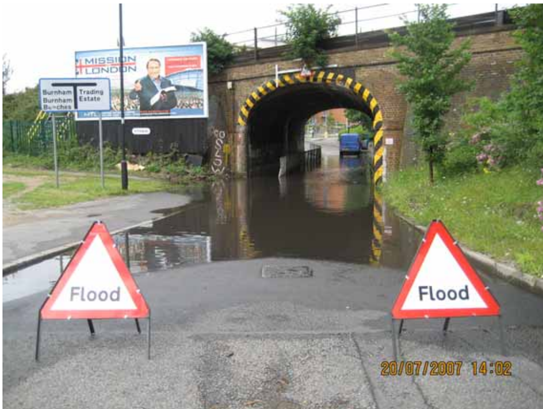
Plate C1 Flooding at railway bridge, Burnham Lane
