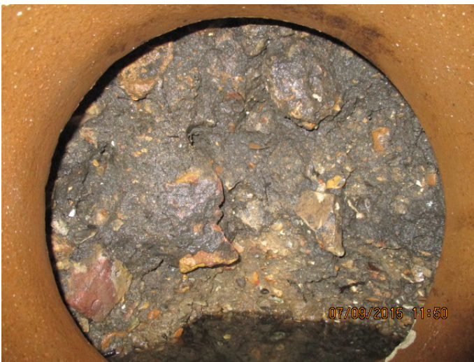
Figure 2-5 Blocked 300mm storm over flow pipe
