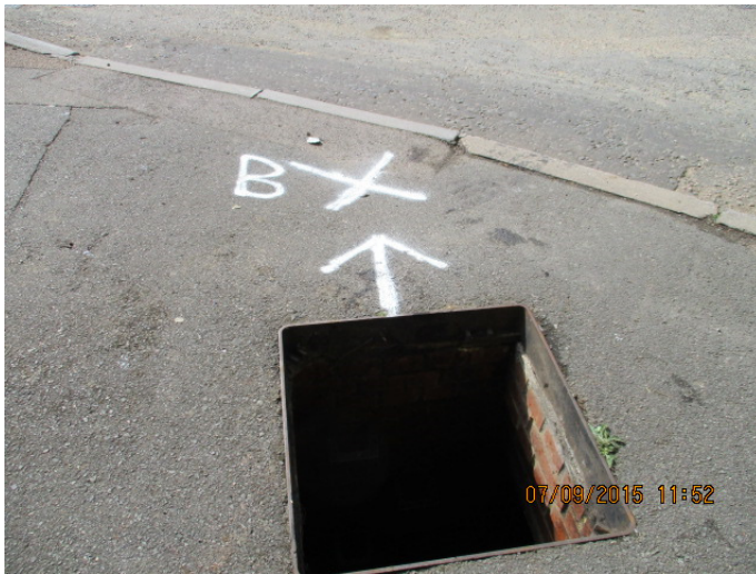
Figure 2-6 Location of blockage, indicated by the white cross (which follows the line of recent utility works)
