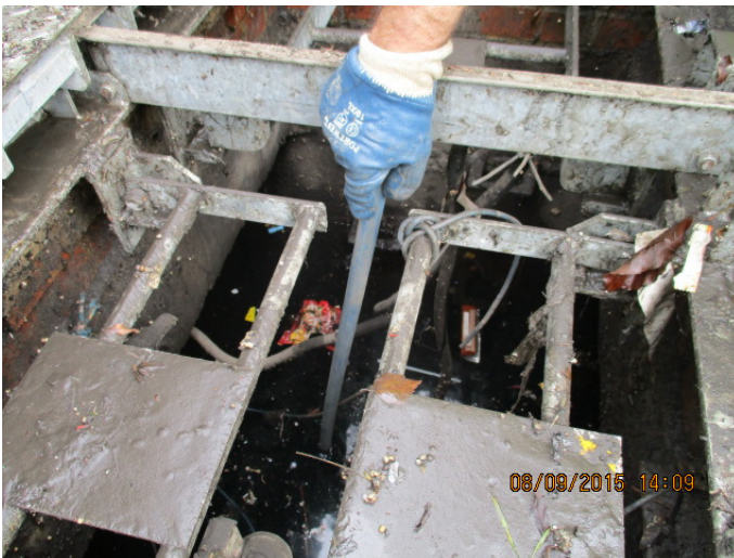
Figure 2-2 Pump station chamber full of water
